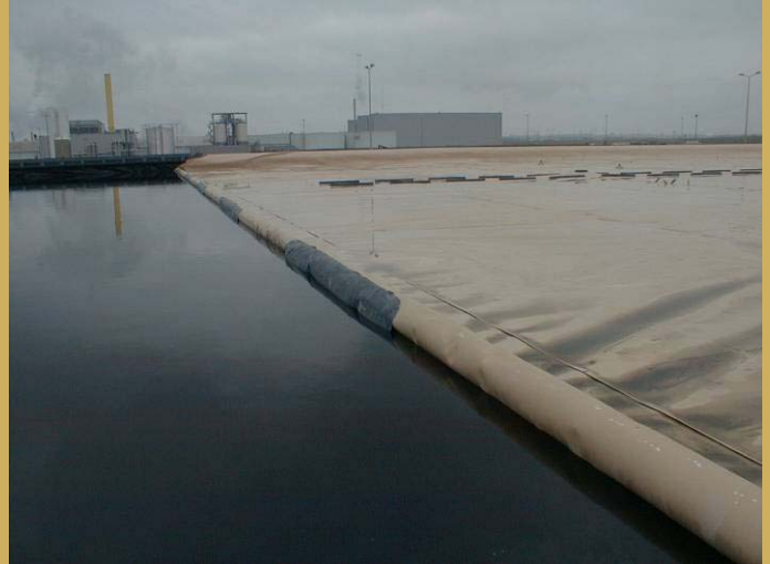
New FLI Geomembrane Cover pulled over full lagoon
