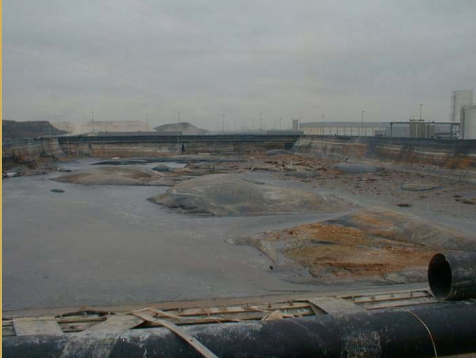
Old Damaged Cover
