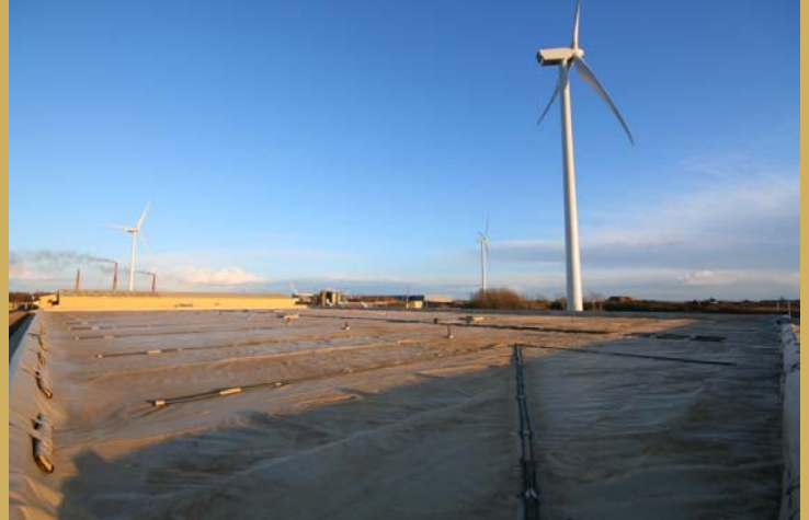
Geomembrane Cover pulled over full lagoon
