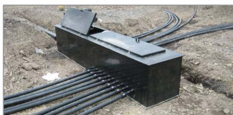
Landfill Gas Manifold
