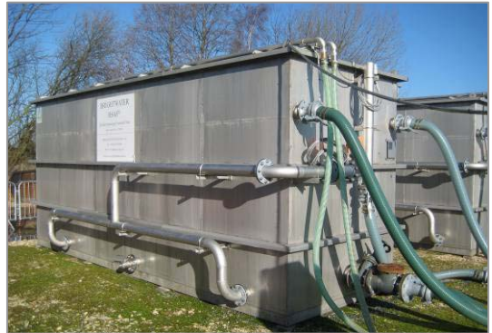
HSAF® units operational on site
