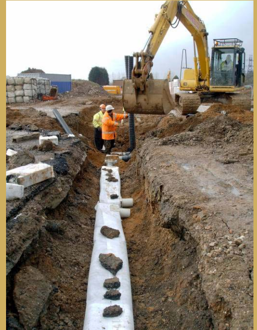
Gas Venting & Dilution Duct
